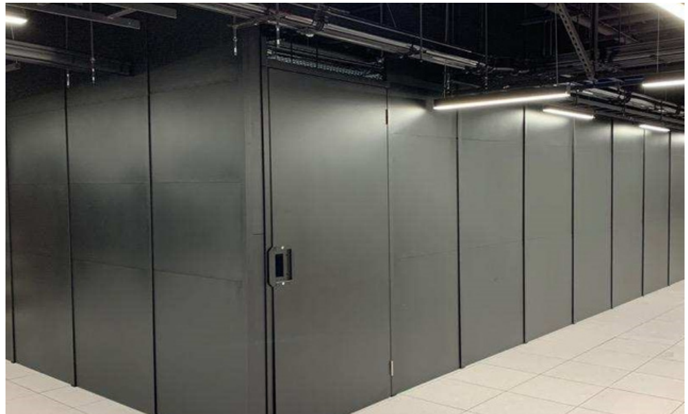
Solid Black Panel with all hardware on the inside of the enclosure.
